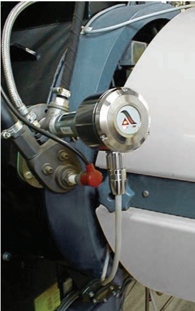
The LAMTEC F200K flame scanner in operation.
